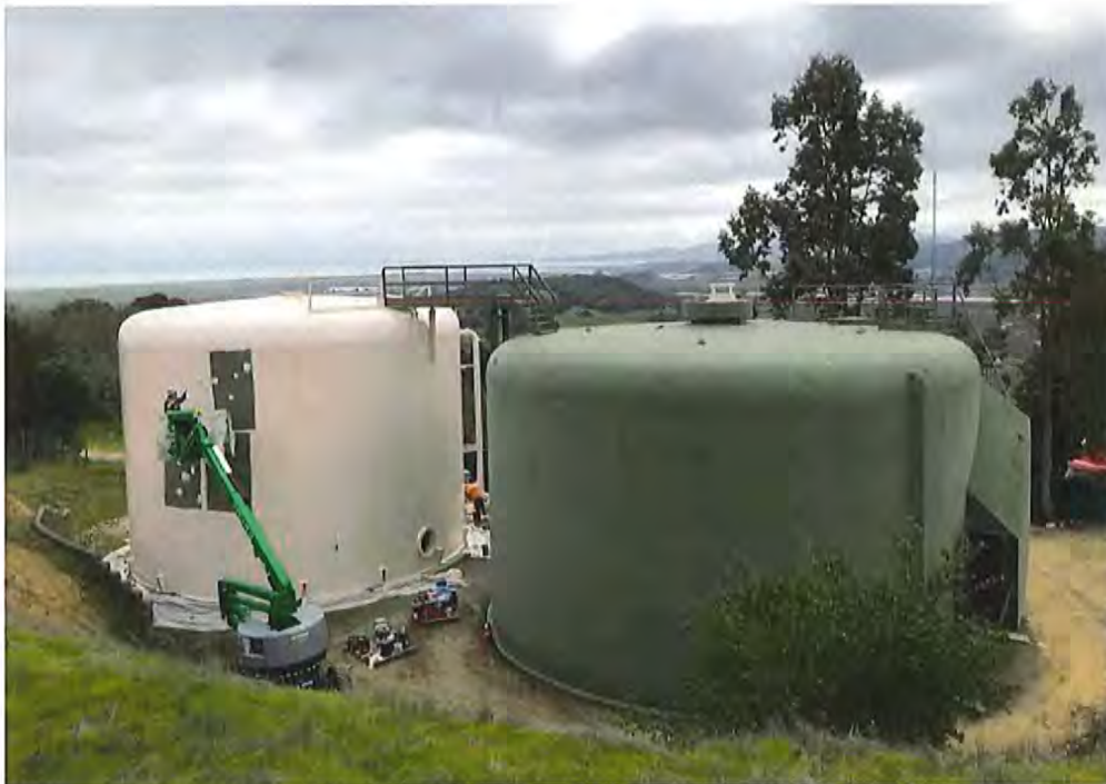
Worker Marcos Mora applies an undercoat paint to a 200,000 gallon water tank in Novato, Calif. on Thursday, Feb. 13, 2020. (Sherry LaVars/Marin Independent Journal)
